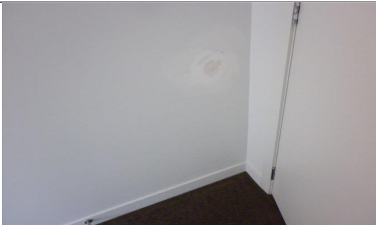
Hole in the wall behind door in third bedroom need finishing.
