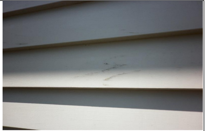
Paint work in need of attention in several areas.
