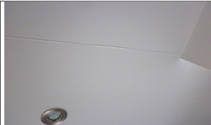
Crack in hall ceiling possibly due to it being a long hallway with no construction joint in the plasterboard. Suggest putting a construction joint in to stop future cracking.
