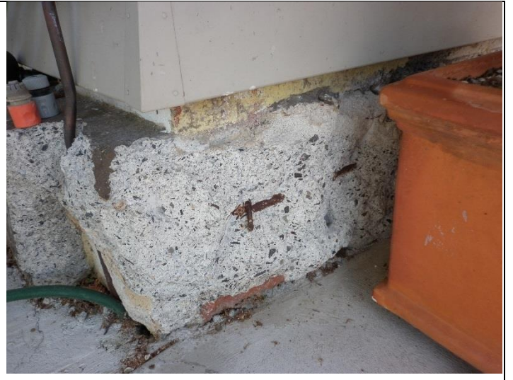
Exposed reinforcing in footing .Suggested plastering over footing to make good and keep steel from further rust.
