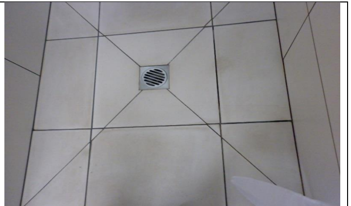
Ensuite tiles require grout to be redone and silicon around the base also needs to be replaced.
